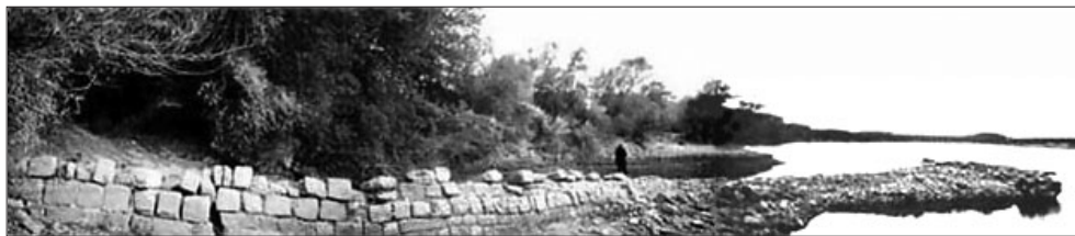
FIG. 3 - Part of the defense wall of the Byzantine Fortress - Ostrov, on the «Păcuiul lui Soare» island, known as Vicina, was initially a military naval base and inhabited until mid-15 th century.
